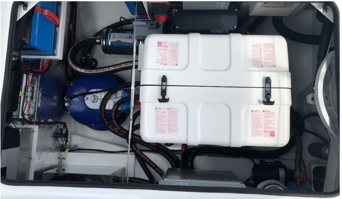
Inside the engine compartment of an Oceanvolt hybrid. The additional sound insulation capsule around the generator plus the normal soundproofing of the compartment means some customers can forget they even have a diesel running!
